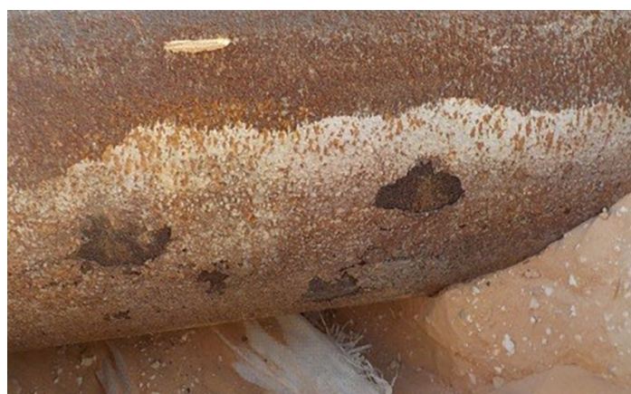
Photos: 1a (above) shows pipe sections covered with sand, 1b (below) shows pipe sections developing pits
